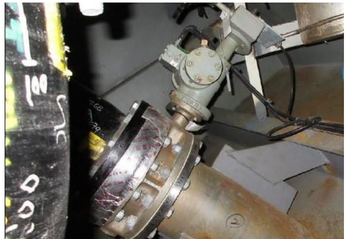
Scrubber overboard discharge connection
